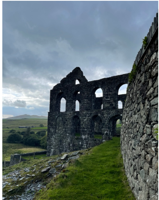
Figure 6e: Photograph of the Ynys y Pandy Slate Mill's outer wall (Own Photography, 2024).
